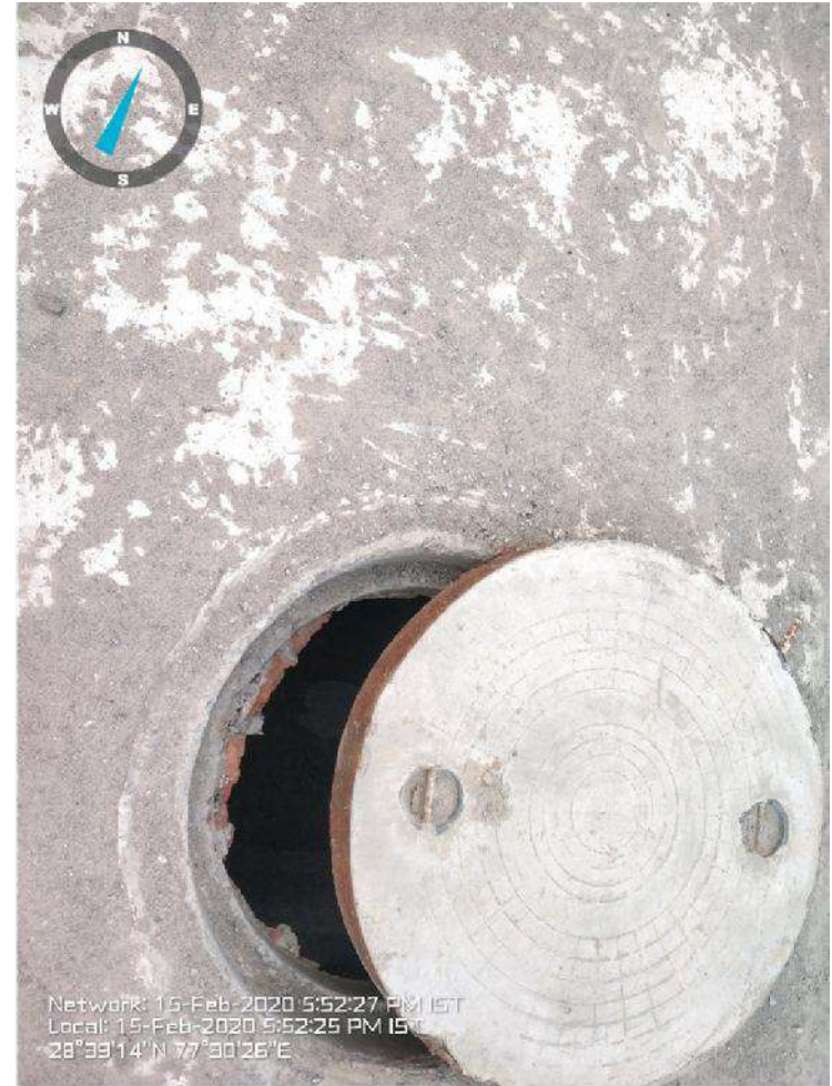
Sec-3 RWH Pit No 1 De Silting chamber in Gallaria
