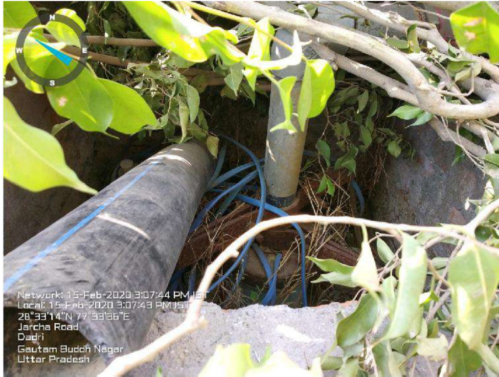
Sec-5 Existing Tubewell in WEF
