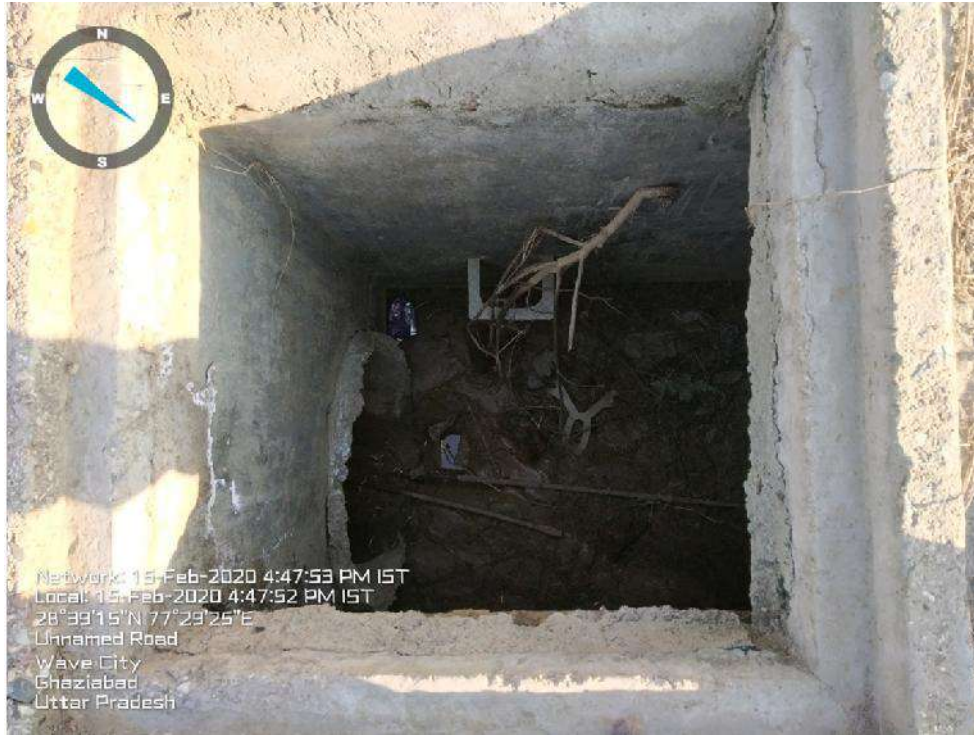
Sec-2 RWH Pit No 18 De Silting Chamber in G-10
