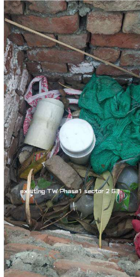
Sec-2 Existing Tubewell 2 in G- 3 Sealed
