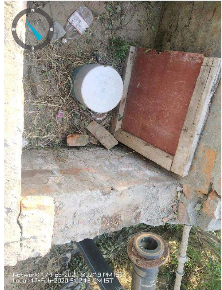
Sec-5 Existing Tubewell in WEF Sealed
