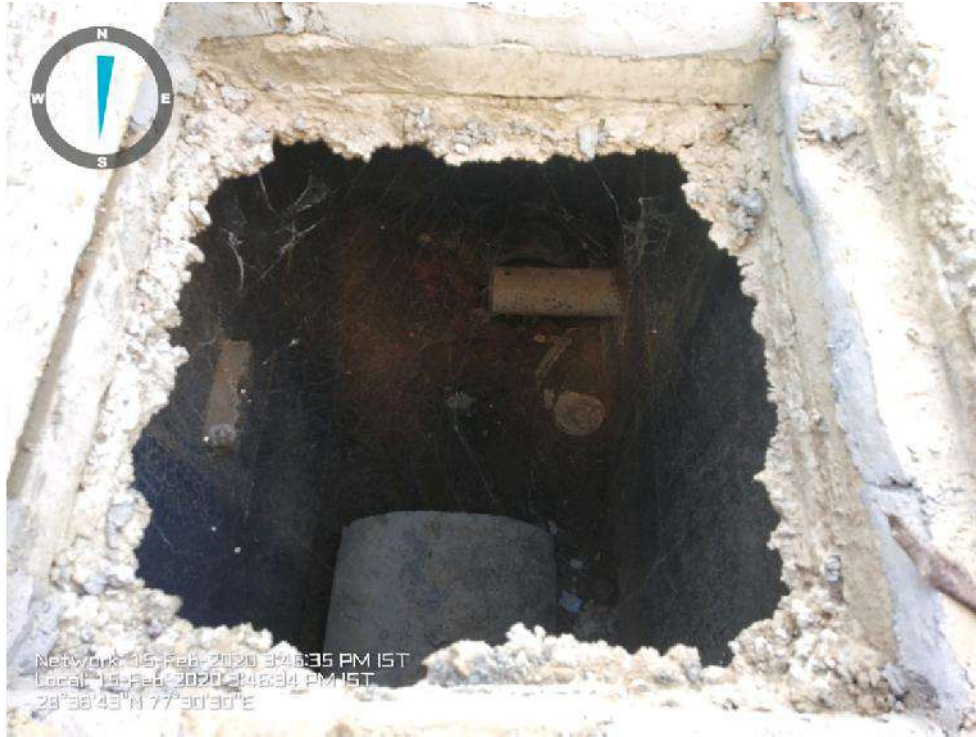
Sec-5 RWH Pit De Silting Chamber in Dream Homes
