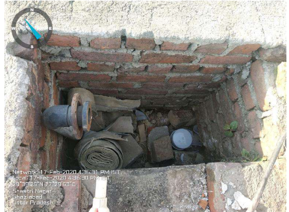
Sec-3 Existing Tubewell in G-22 Sealed
