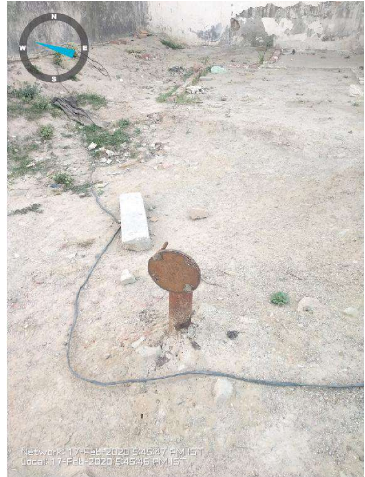
Sec-2 Existing Tubewell 1275 Sealed
