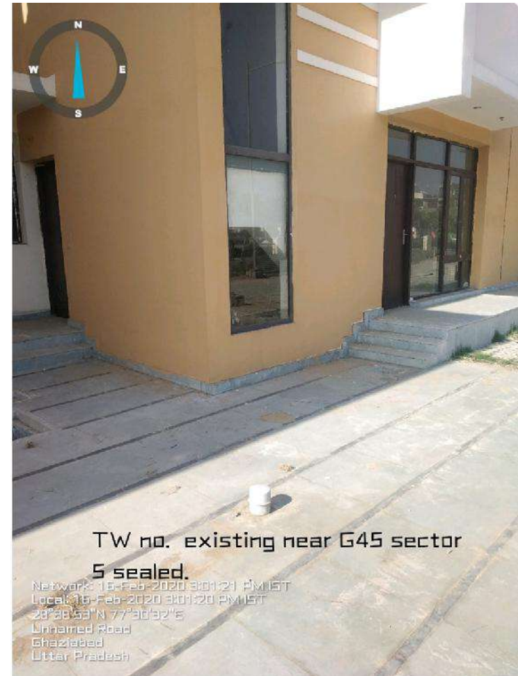
Sec-5 Existing Tubewell 1060 Sealed
