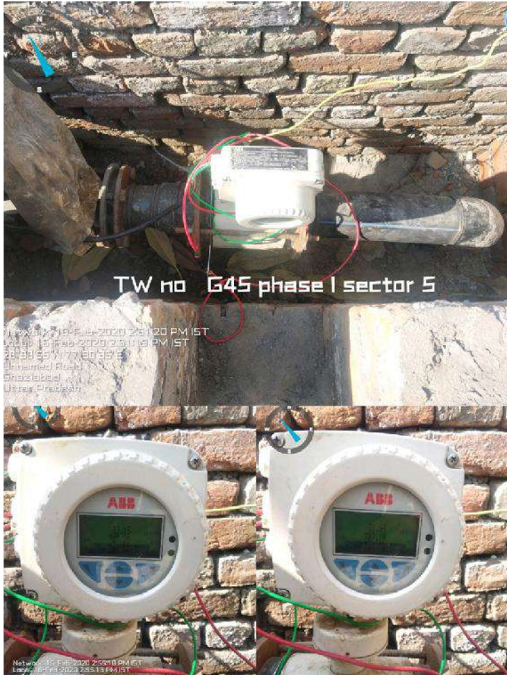
Sec-5, Flow meter at Tubewell at G-45
