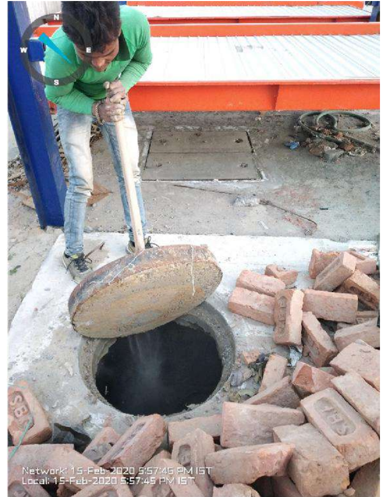
Sec-3 RWH Pit No 2 De Silting Chamber in Gallaria
