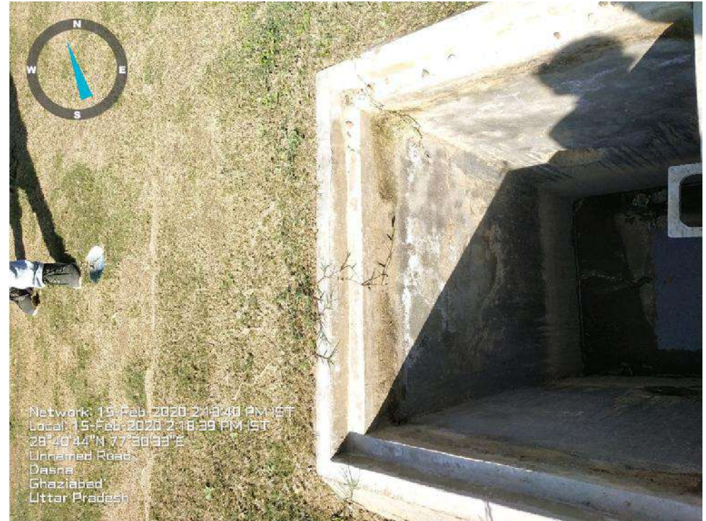
Sec-5 RWH Pit No 9 De Silting Chamber in WEF
