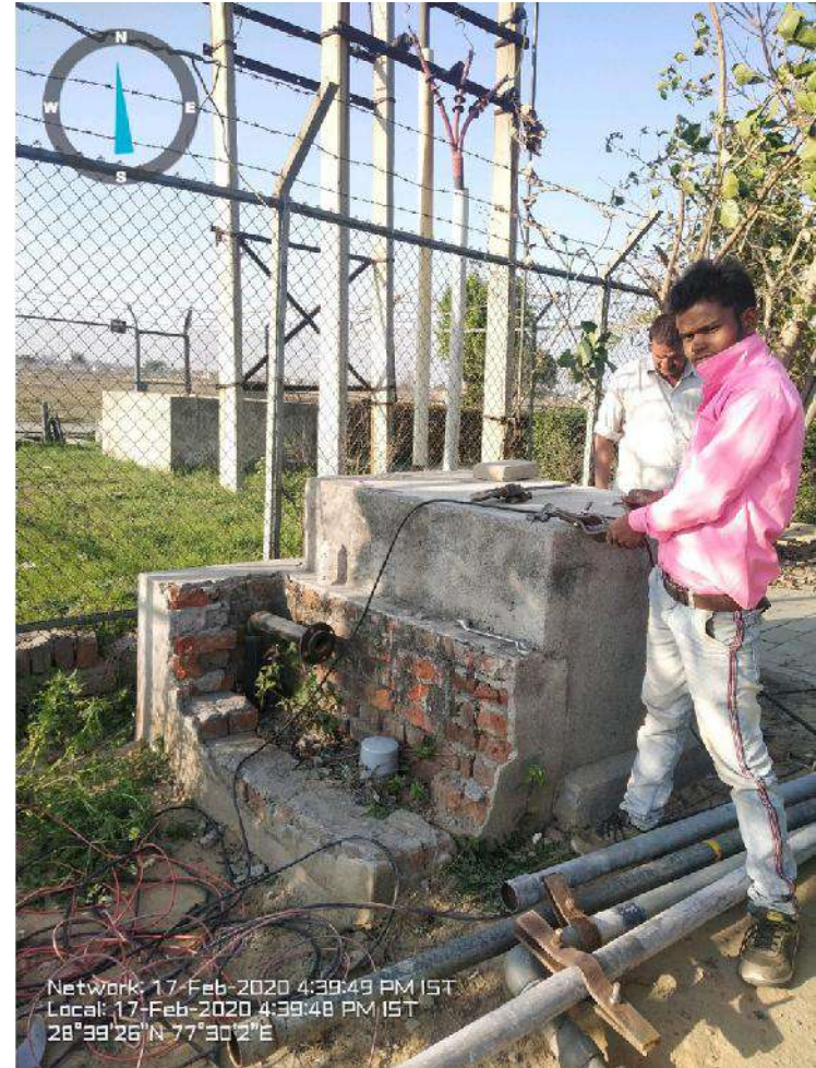
Sec-3 Existing Tubewell G-24 Sealed
