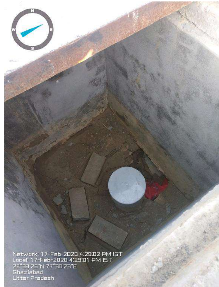
Sec-3 Existing Tubewell in G-28 Sealed
