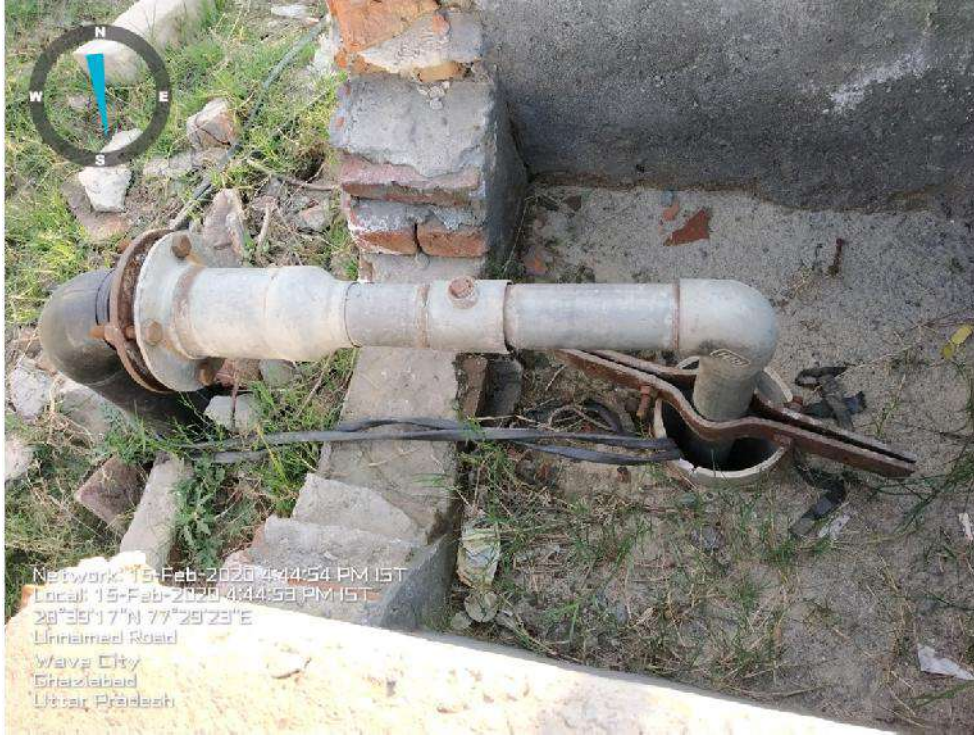
Sec-2 Existing Tubewell at G-10
