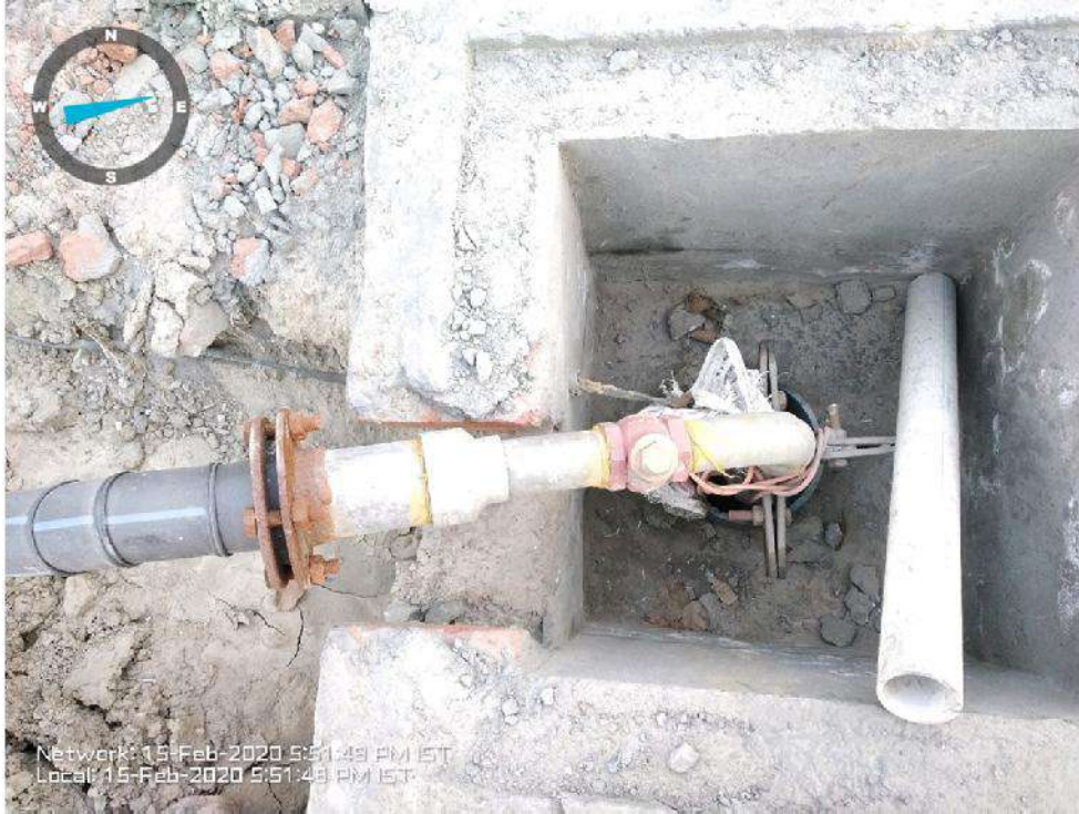
Sec-3 Existing Tubewell 2 in Galleria
