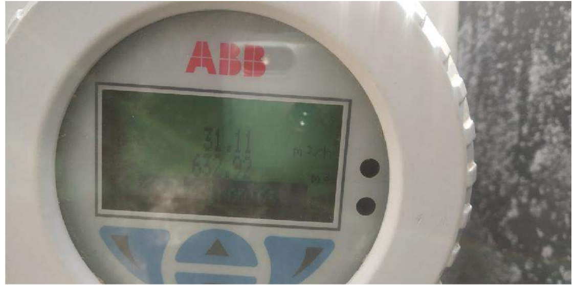
Sec-5 Flow Meter at Tubewell in WEF
