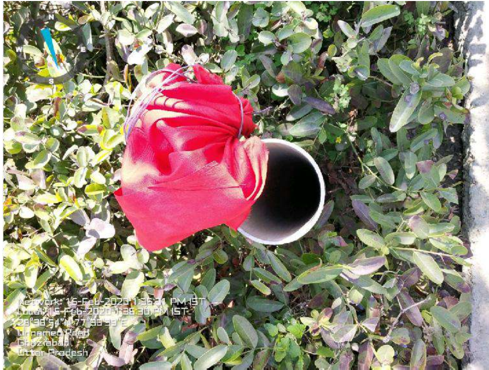
Sec-5, Existing Tubewell at G-42
