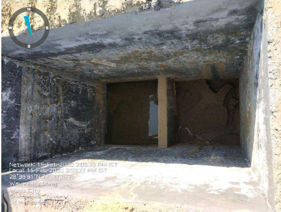
Sec-5 RWH Pit 7 De-Silting Chamber in G-32
