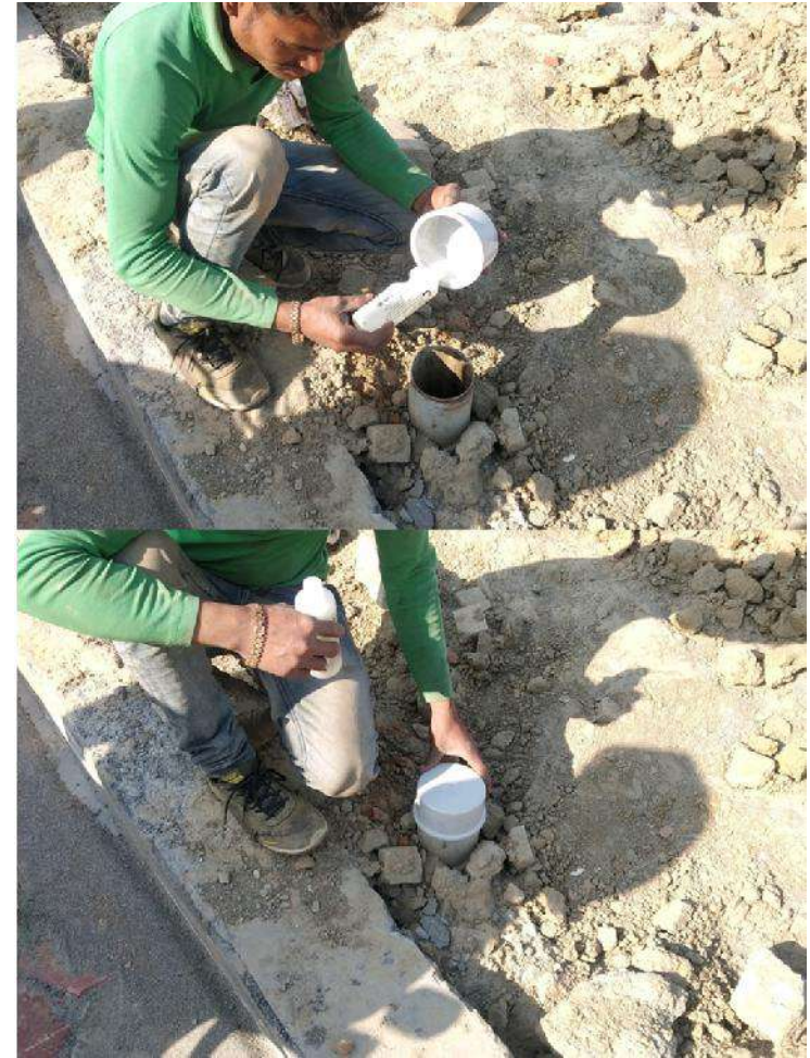
Sec-5 Existing Tubewell G-37 Open and Sealed
