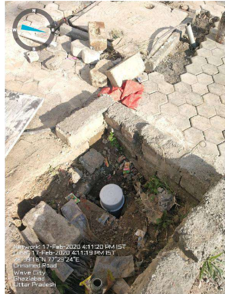
Sec-2 Existing Tubewell 990 Sealed
