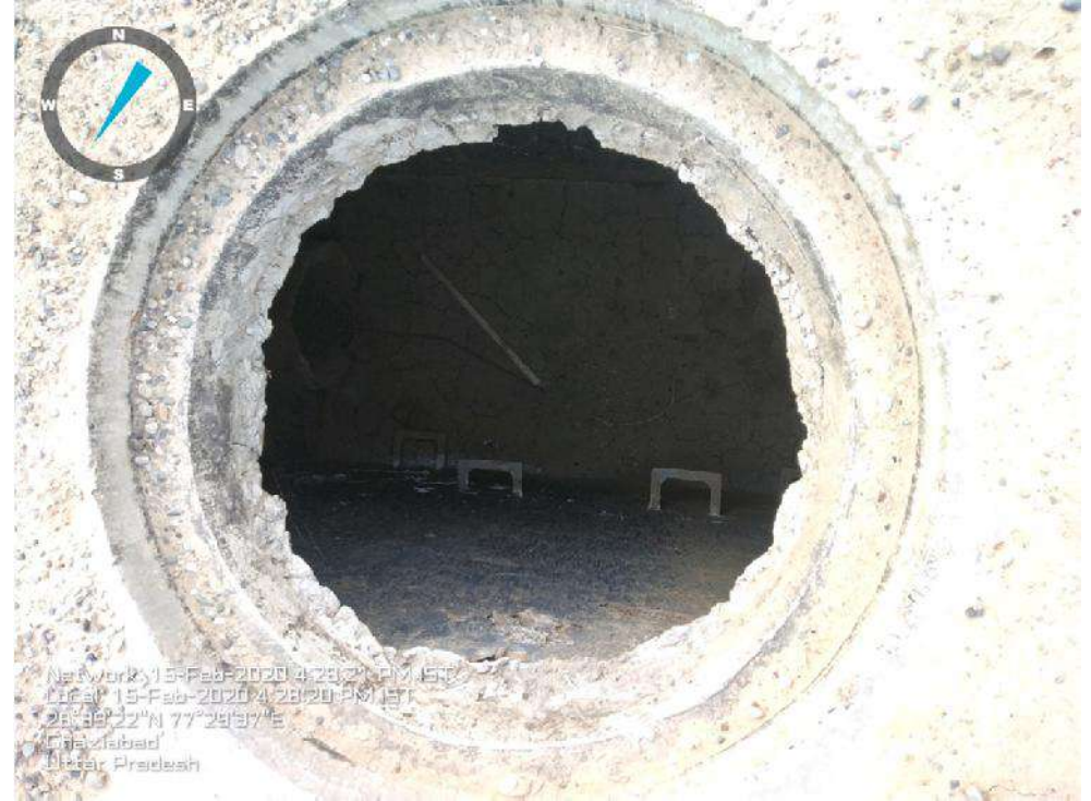
Sec-2 RWH Pit no 15 De Silting chamber in G-5
