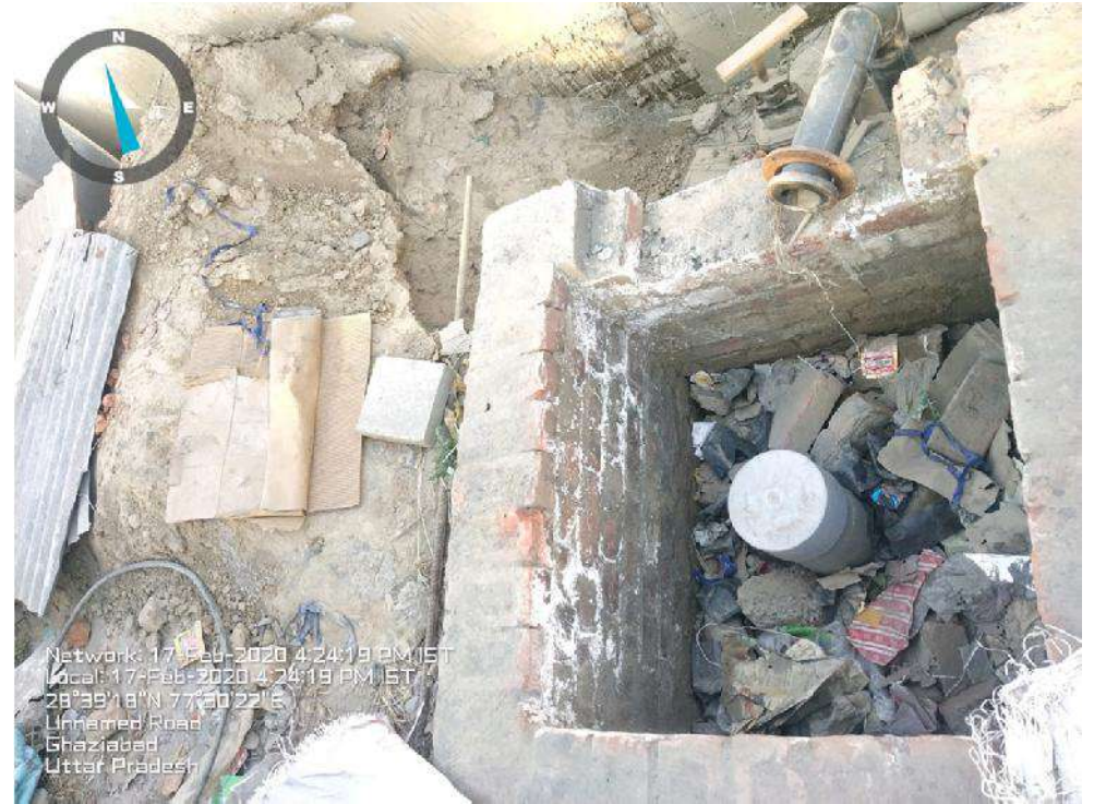
Sec-3 Tubewell 1 Galleria Sealed
